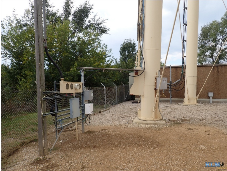
Photo No. 43 View of electrical equipment and mounts
