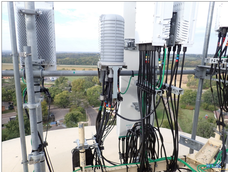
Photo No. 20 View of antennas
