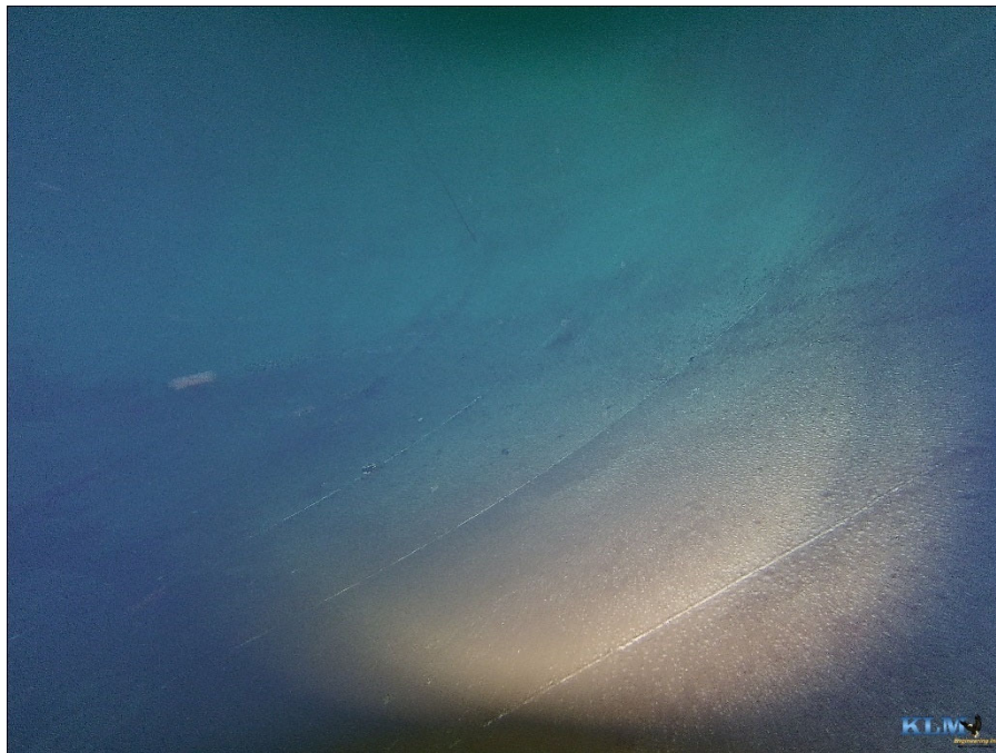
Photo No. 12 Lower torus coating conditions
