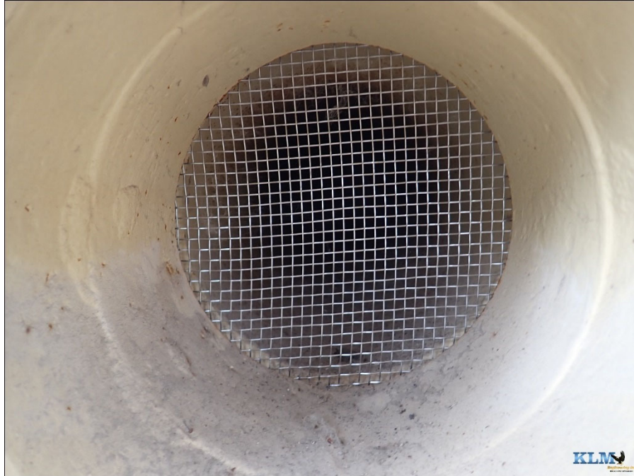
Photo No. 51 Overflow pipe screen
