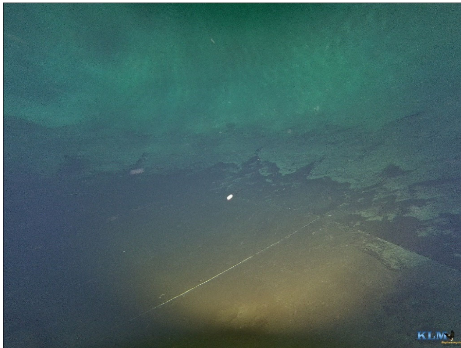
Photo No. 14 Lower torus and bowl coating conditions
