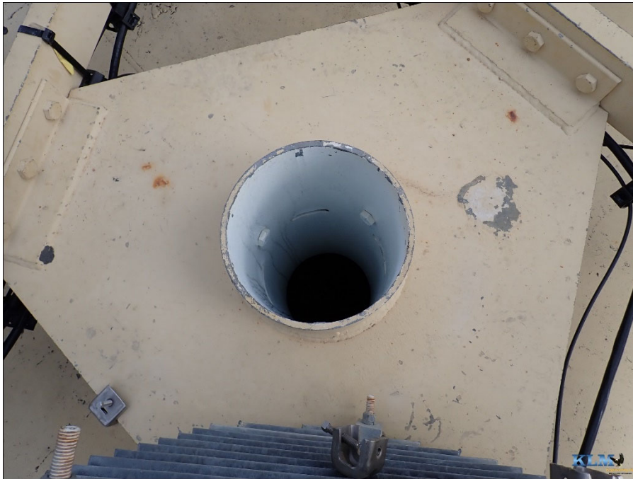
Photo No. 24 Vent collar and platform
