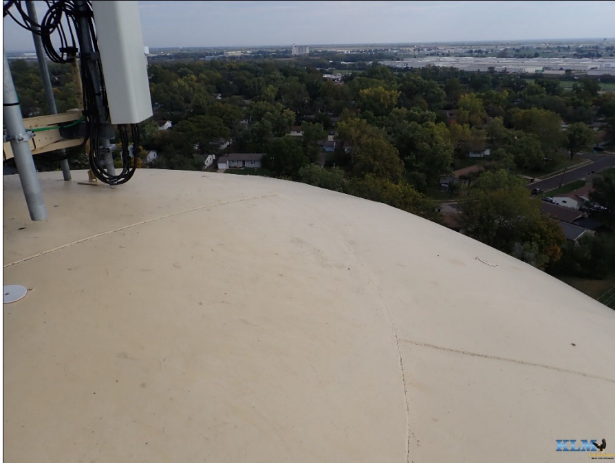
Photo No. 31 View of roof and upper torus Cathodic protection system handholes visible
