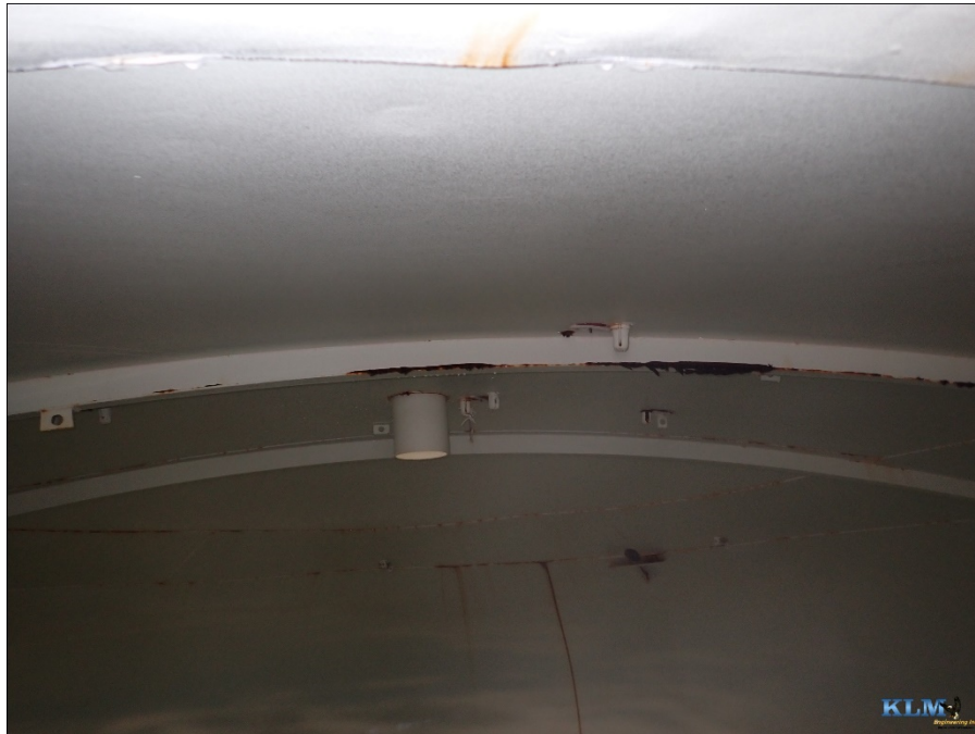
Photo No. 2 View of interior wet roof and stiffeners Vent collar and CP handholes visible
