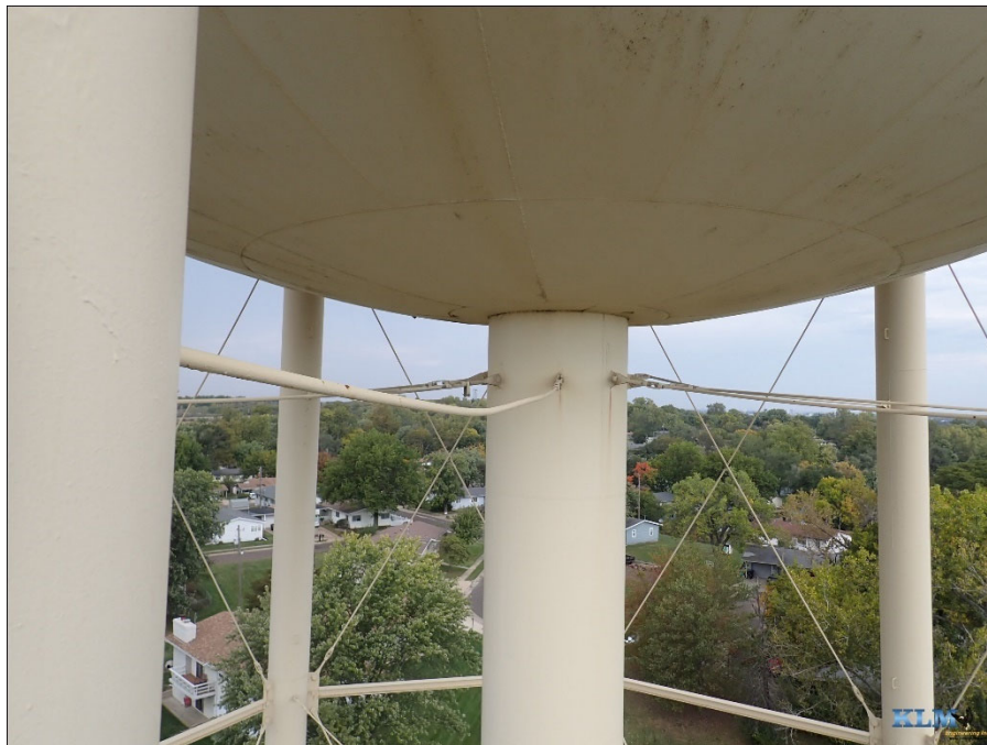
Photo No. 38 Wet riser to bowl connection
