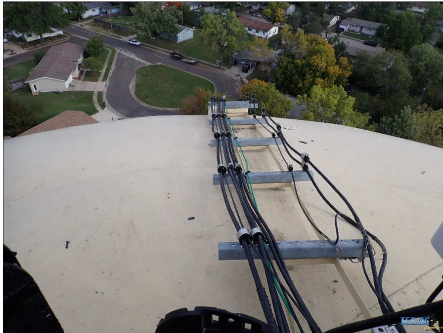
Photo No. 26 Cable mounting brackets
